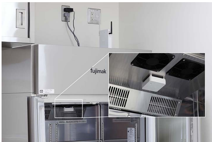
Kitchen Link Cloud sensor installed in SHIMA's refrigerator-freezer (zoomed-in photo) and the parent unit for communication (top of the refrigerator)
