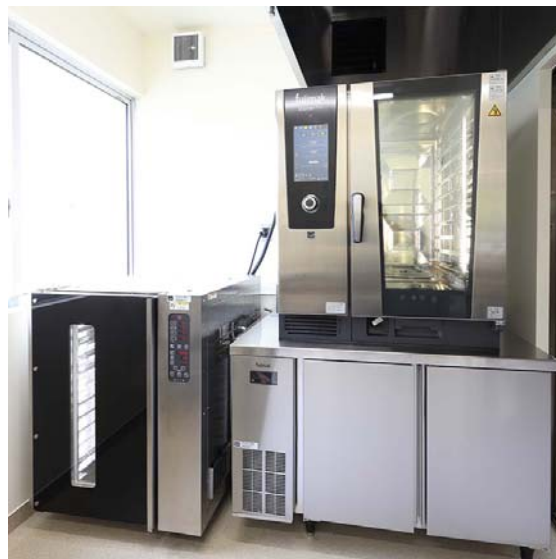
Bread-making area In addition to a combi oven and a table-type refrigerator/freezer, they also installed a dough conditioner that controls fermentation at every stage, from frozen dough to scratch dough.
