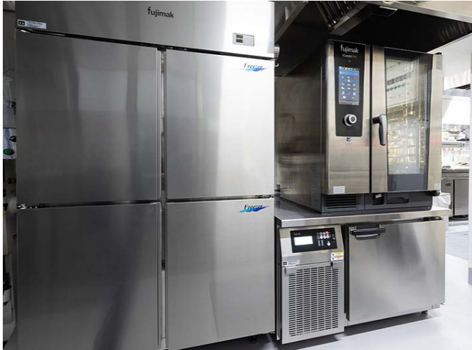
A blast chiller is installed under the combi oven. "We can remove the food from the oven and start rapid cooling right away," Chef Takayama says.
