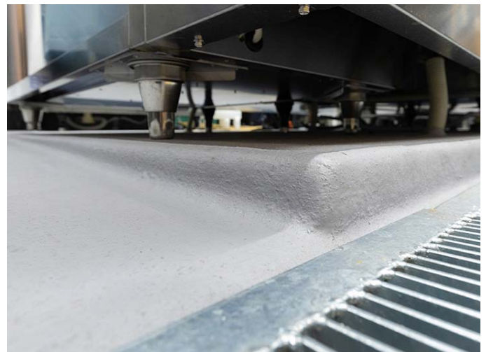
The floor is coated with water-resistant FRP paint with grating that is sloped to allow for drainage when cleaning.
